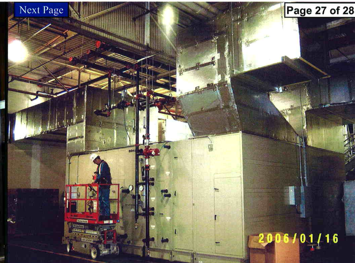
Crankshaft Dept. – AHU w/ Piping Connections
